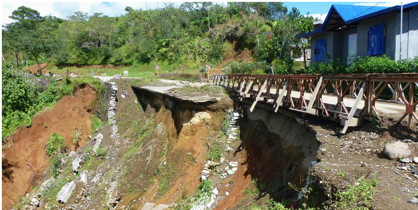
Landslide and road damage in the Philippines. Source: Tunatura/Shutterstock
